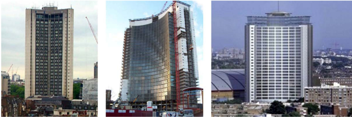
Fig. 6. Vertical and horizontal extension to the Empress State Building using braced steel framing.
